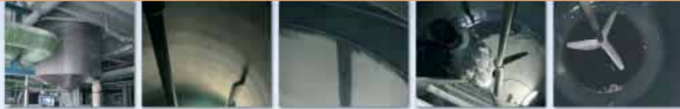
Mechanical removal of rusted patches and drying of inner surface Abrasive blast to surface profile of 75 µm and surface cleanliness SA 3 Application of Loctite® 7227 on weld lines Full surface coated, then after partial cure the second coat was applied After 24 hrs, the tank was ready to be filled
