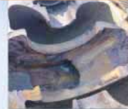
Pic. 1: Corrosion and erosion were clearly evident
