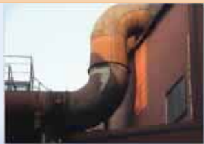
Coke Plant Pipe Elbow
