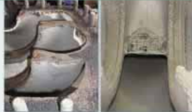
Pitting and erosion was clearly evident
