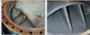
The corroded butterfly valve – before and after repair
