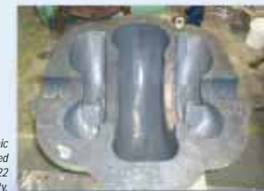
Loctite® Nordbak® 7227 Brushable Ceramic Grey applied to seal the blast. Fill the corroded and abraded areas using Loctite® Wear 7222 Resistant Putty
