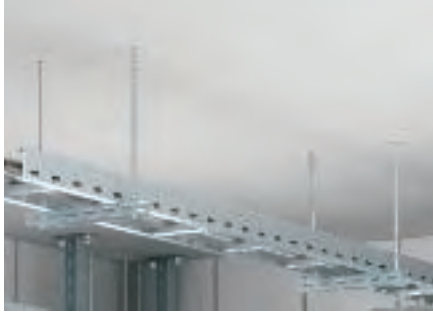
Suspension of a cable ladder with threaded rods and U supports as a cross-section.
