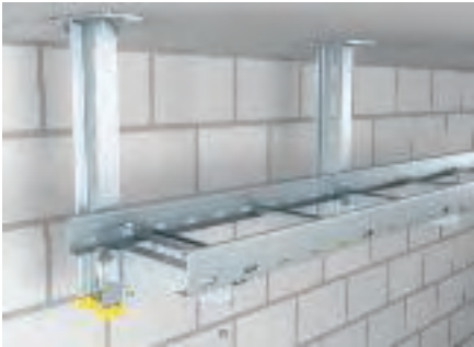
Suspension of a cable ladder with supports and support brackets.
